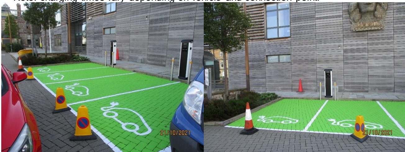
Images of free standing dual EV charging units, with marked parking bays, installed at Helensburgh and Lomond Civic Centre
